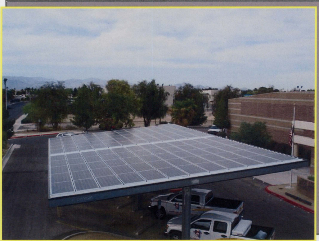
Figure 1: Example of a carport photovoltaic system
