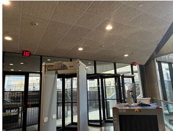
Figure 7. Means of Egress Doors with Exit Signs 27
