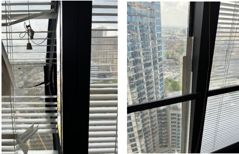
Figure 8. Damaged Window Seals in Office Space 31
