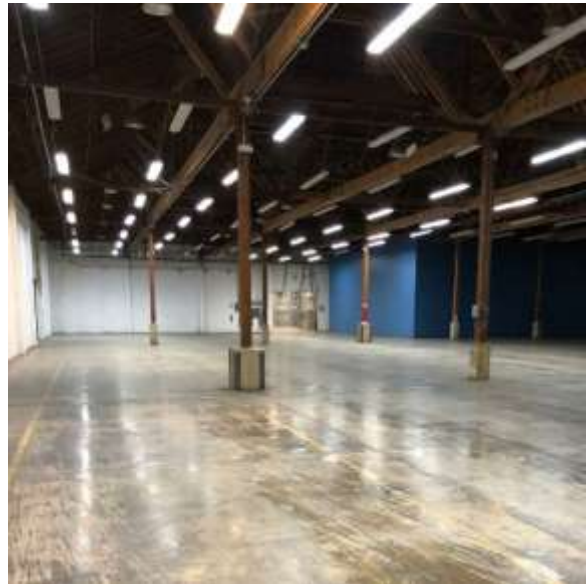
Image 4 - Tenant vacated this space in May 2023
