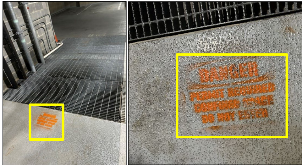
Figure 2. Illegible Permit Space Label Near a Sewage Ejector Pit at the Elijah Barrett Prettyman U.S. Courthouse 10
