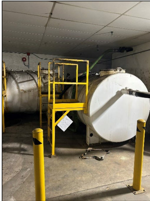
Figure 5. Unlabeled Grease Traps at the Richard B. Russell Federal Building and U.S. Courthouse 13
