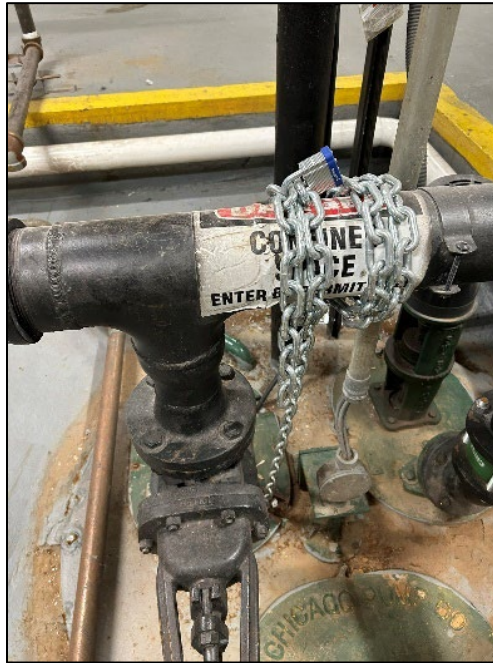
Figure 6. Obstructed Permit Space Label on a Sump Pump Pit at the Elbert P. Tuttle U.S. Court of Appeals Building 15
