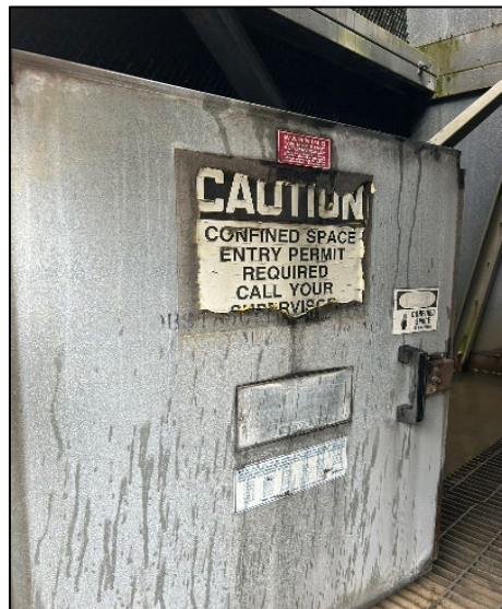
Figure 7. Faded and Damaged Permit Space Label on a Cooling Tower at the Richard B. Russell Federal Building and U.S. Courthouse 16
