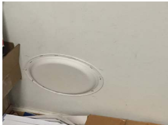
Figure 4: Paper plate used to repair hole in the wall.
