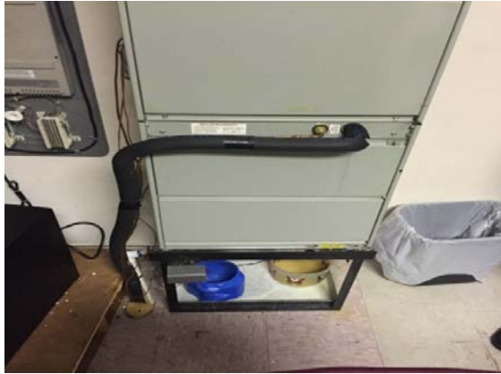
Figure 1: HVAC unit with make-shift water collectors.
