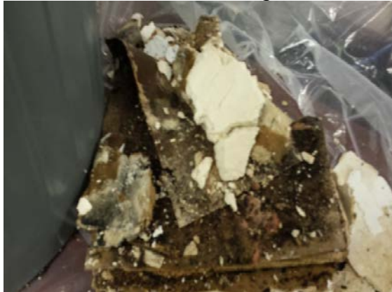
Figure 5: Section of drywall ceiling that fell in the third floor training room.
