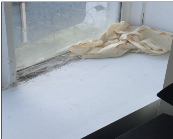
Figure 3: Unsealed leaking window.
