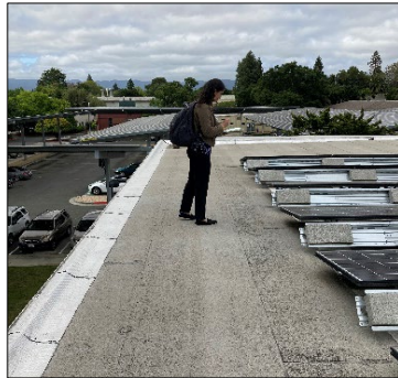
Figure 2 – Panels Next to Roof Edge without Fall Protection (Person for Scale)
