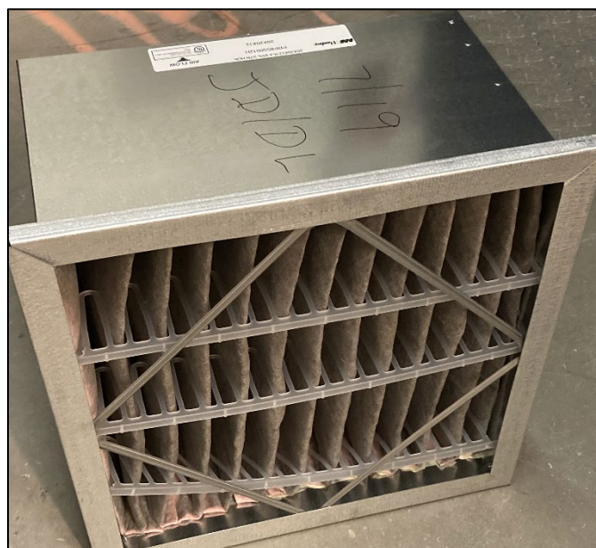
Figure 5 – Air Filter in Operation at the Mary E. Switzer Federal Building, Washington, D.C. 13
