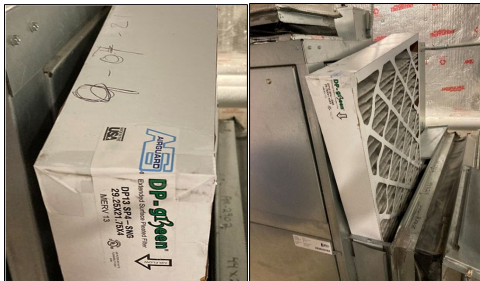
Figure 7 – Air Filter in an AHU at the HHS Parklawn Office Building, Rockville, Maryland 15
