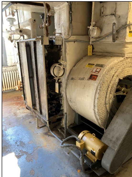
Figure 1 – AHU in the GSA Headquarters Building, Washington, D.C. 9
